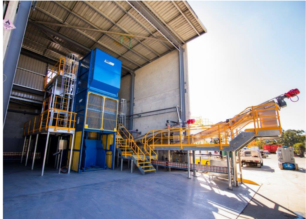
Hazpak paint de-packaging unit
